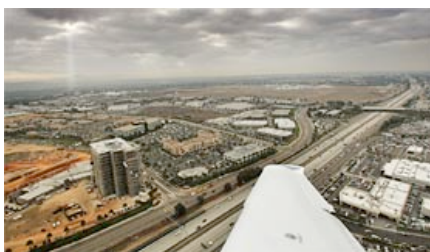
HOWARD LIPIN / Union-Tribune Some pilots say Sunroad Enterprises' 12-story office tower under construction, seen in the lower left corner of this aerial photo, presents a hazard during bad-weather landings at Kearny Mesa's Montgomery Field, which is visible at the top of the photo.
