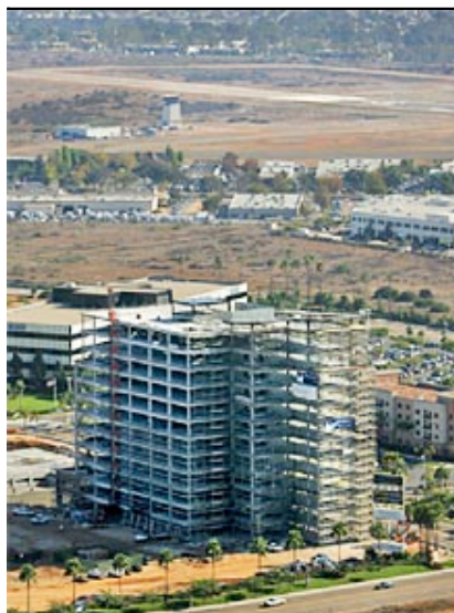
HOWARD LIPIN / Union-Tribune The FAA has declared this 12-story building under construction near Montgomery Field a hazard.
