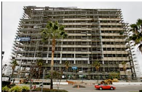
HOWARD LIPIN / Union-Tribune Federal, state and city officials continue to battle with the developer over the height of the 12-story Sunroad Centrum office building under construction near Montgomery Field.
